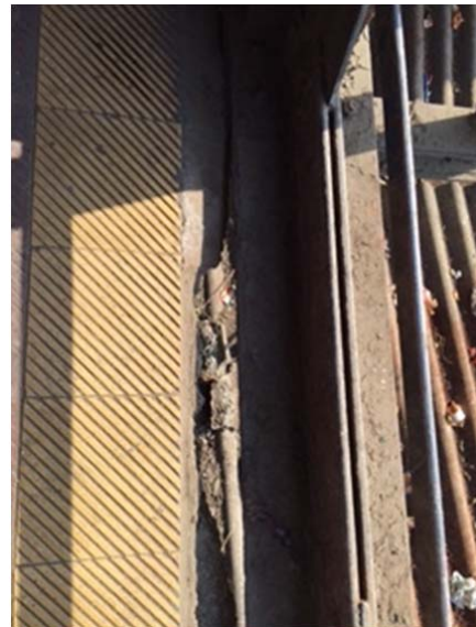
Figure 9: Gaps on the corners of FOBs
