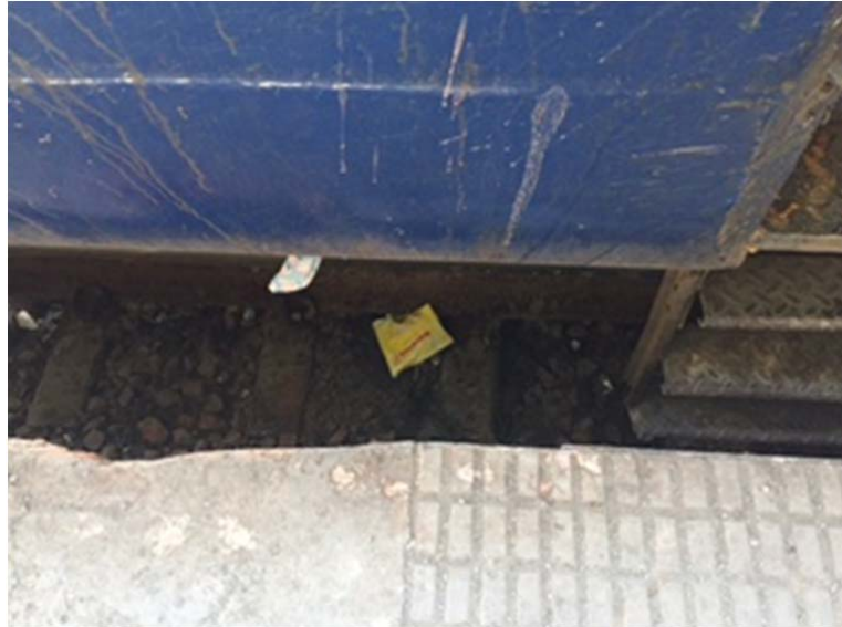
Figure 8: Platform gap on platform 5
